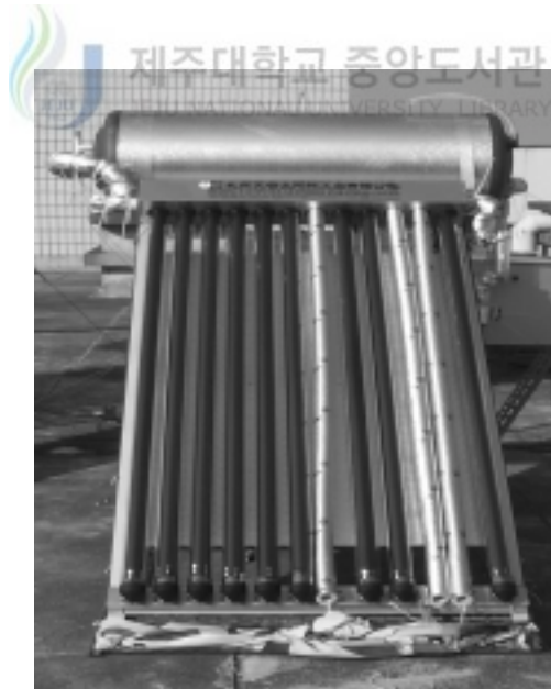
Fig. 16 Photograph of the installed 10mm U-pipe type system
