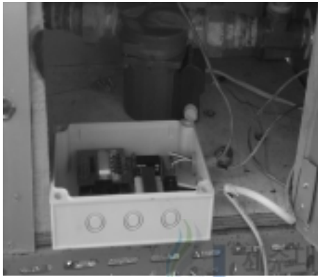
Fig. 10 Photograph of the differential temperature controller and the pump
