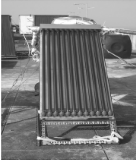
Fig. 15 Photograph of the installed 8mm U-pipe type system
