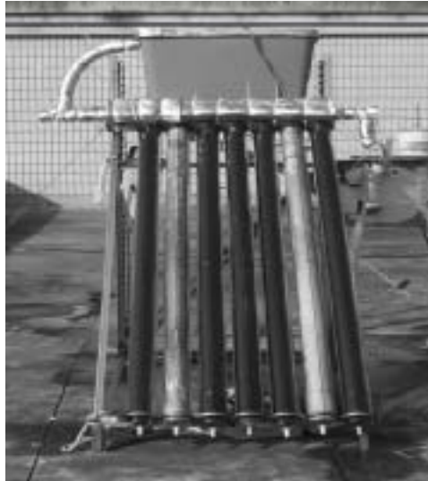
Fig. 17 Photograph of the installed single vacuum tube system with heat pipes(SEIDO 5)
