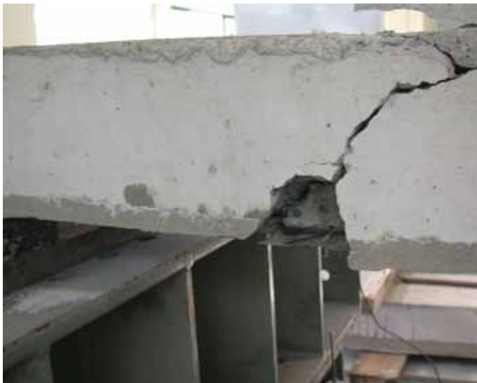
Fig 4.16 CFRP grid dowel rupture(C4A-2T-2)
