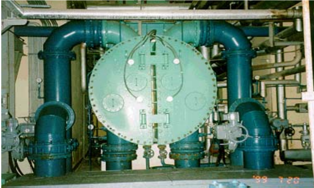
Fig. 10 Condenser system of Bukcheju thermal power plant No.1 unit
