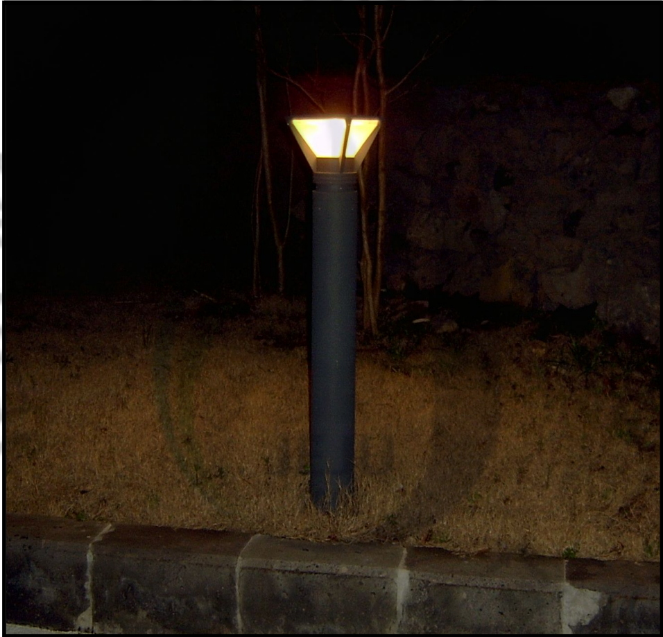
Fig. 3 Installed luminaire of bollard type
