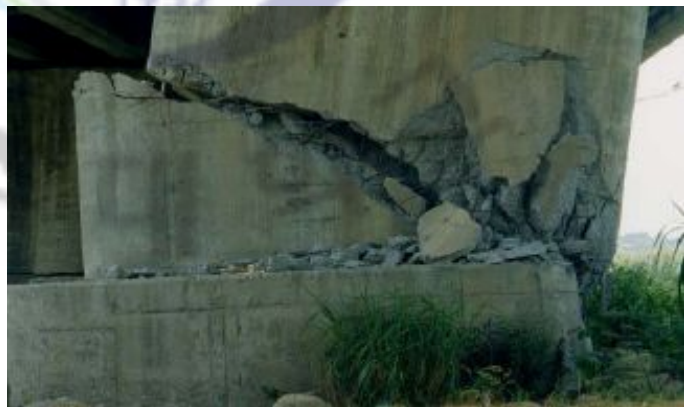
(b) 1999 Earthquake in Taipei
