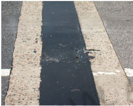
(a) Tensile failure or pitting
