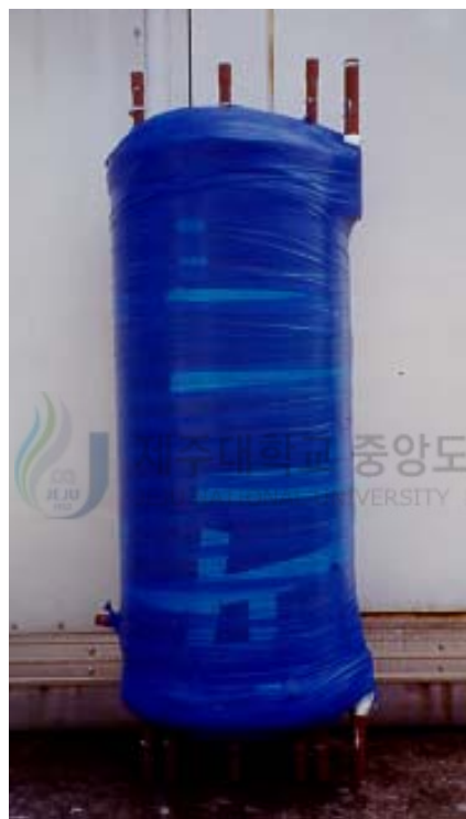
Fig. 4 Insulated storage tank
