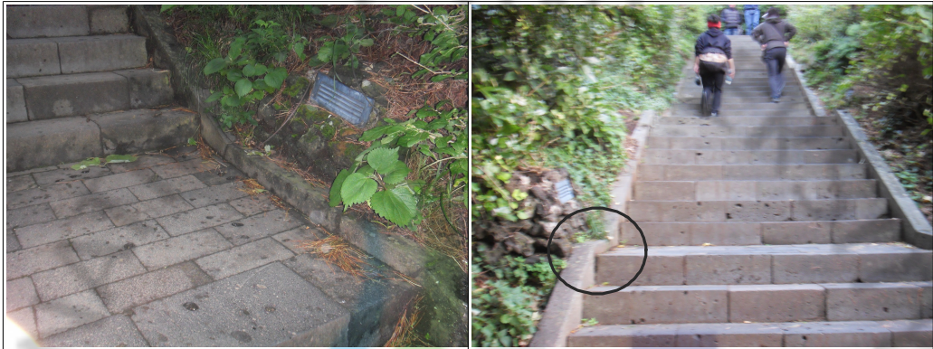
Fig. 6 External appearance of installed luminaire at the stairs section
