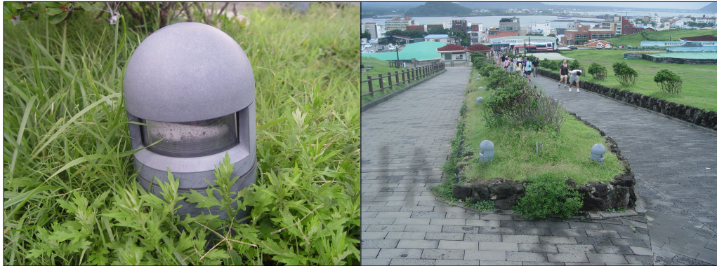
Fig. 2 External appearance of installed luminaire at flower bed
