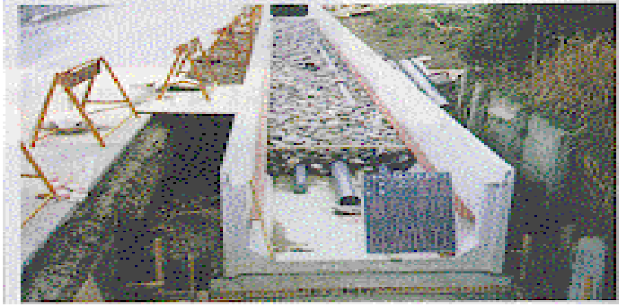
Fig. 4-10. Examples of installation of gravel contact oxidation waterway as drainage into waterway
