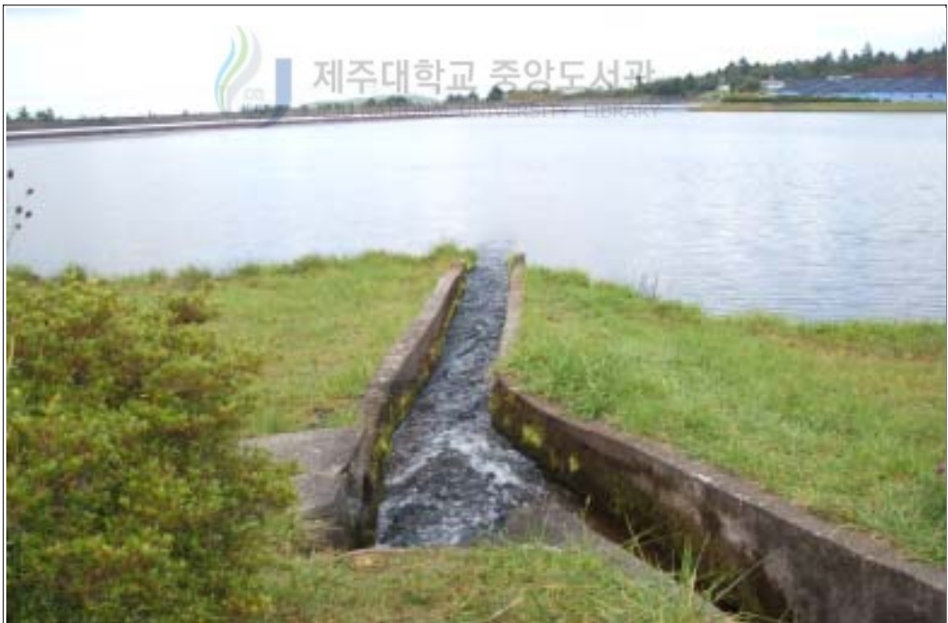
Fig. 4-13. The overall view of the water canal of the inlet of Eoseungsaeng dam
