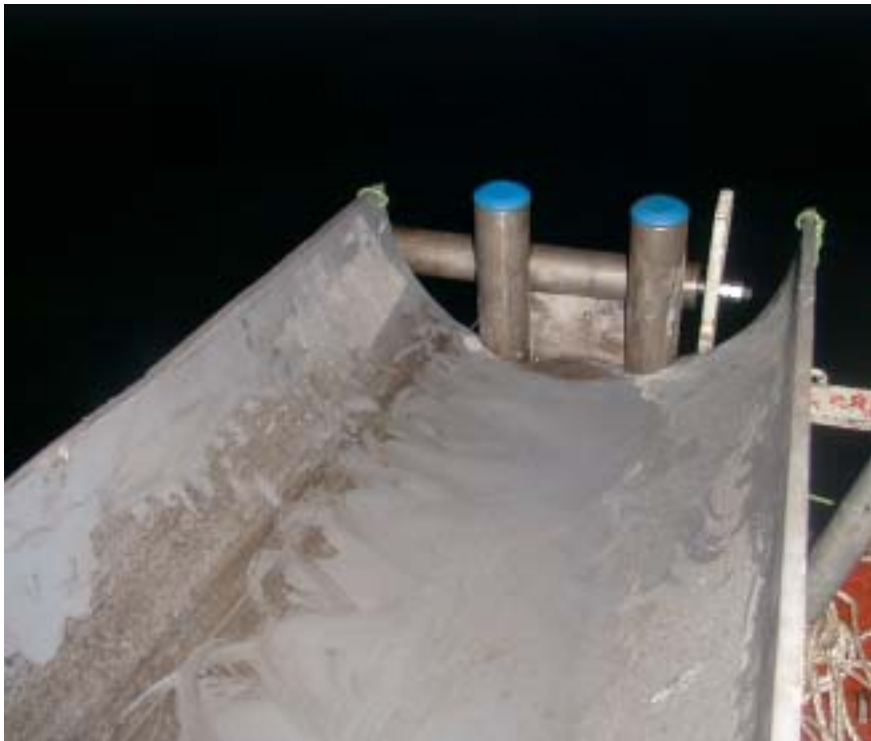
Fig. 14. The linking of side roller and inducement tube equipment of the main line.
