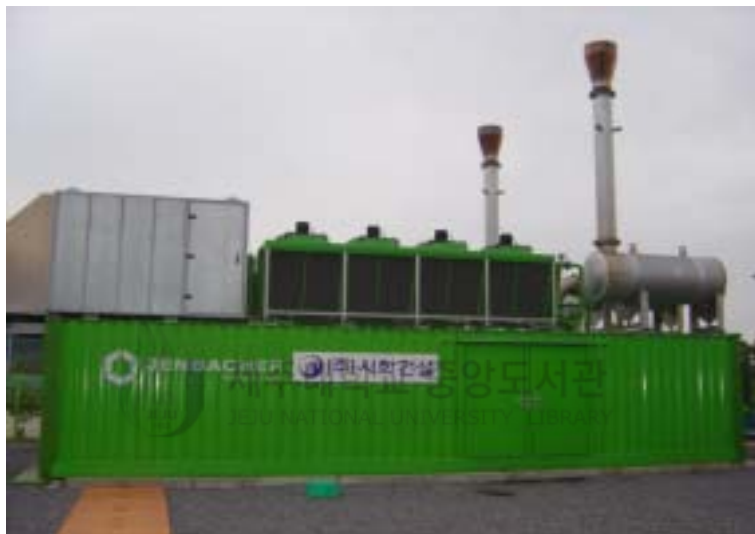
Fig. 2-6 View of the LFG Power Plant
