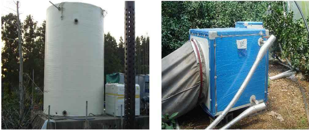
Picture 3-5 The heat tank and fan-coil unit
