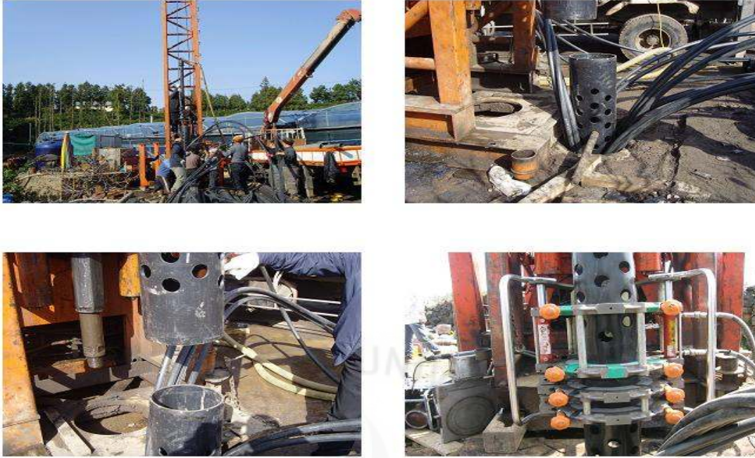
Fig. 3-3 The installation of the circulating loop for water loop
