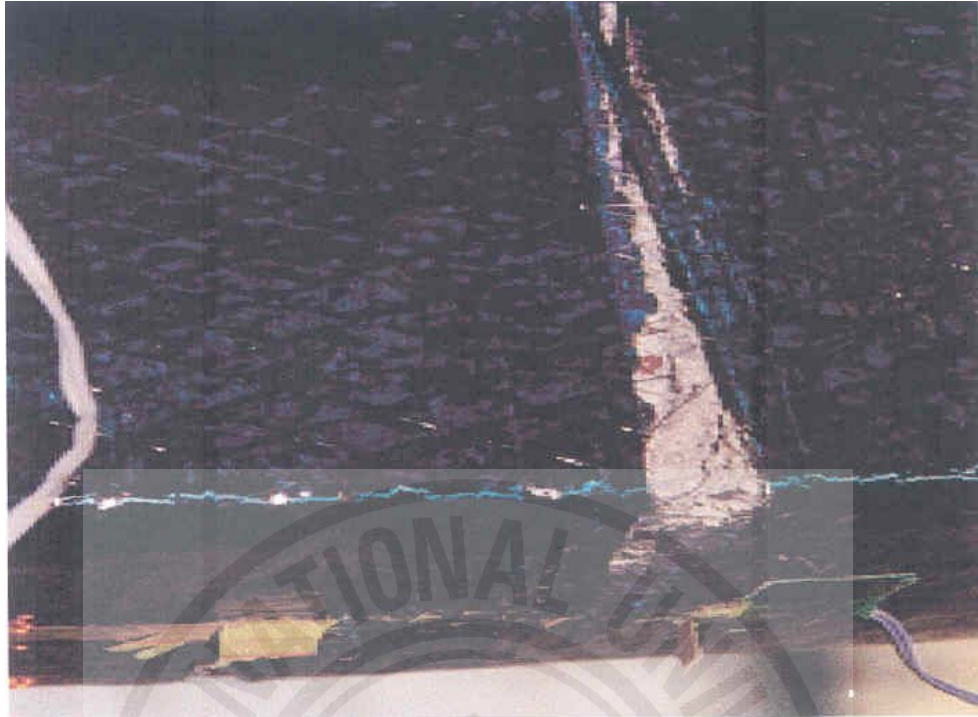
Fig. 4.20 Tensile failure of CFRP sheet (F2W)
