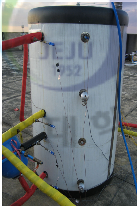
Fig. 2-3 Picture of the thermal storage tank
