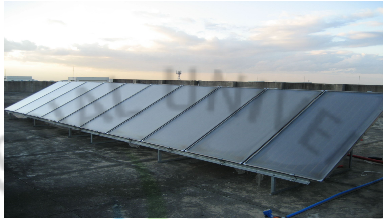
Fig. 2-1 Picture of solar collectors
