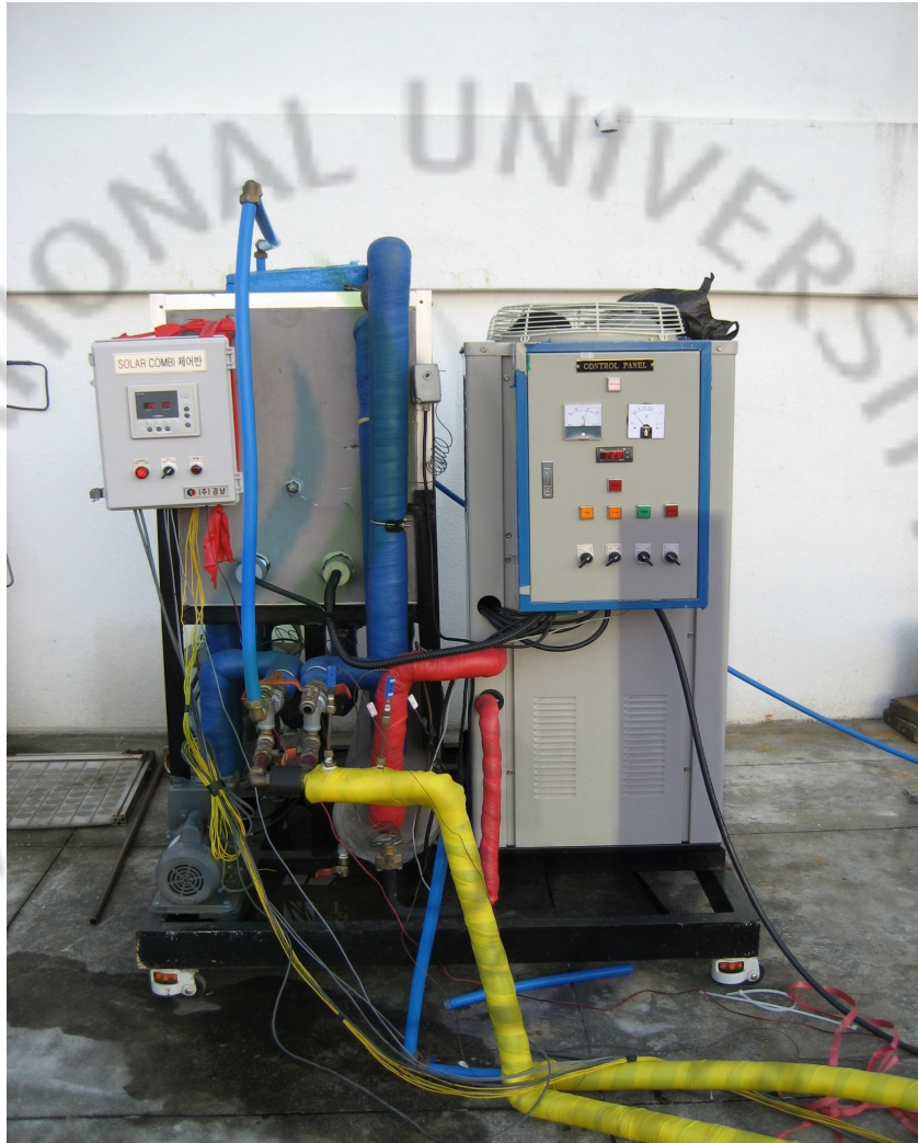
Fig. 2-13 Picture of system controller and chiller controller
