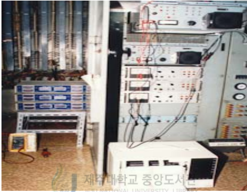
Fig. 22 Experimental test station using a proposed backup system in Pukcheju
