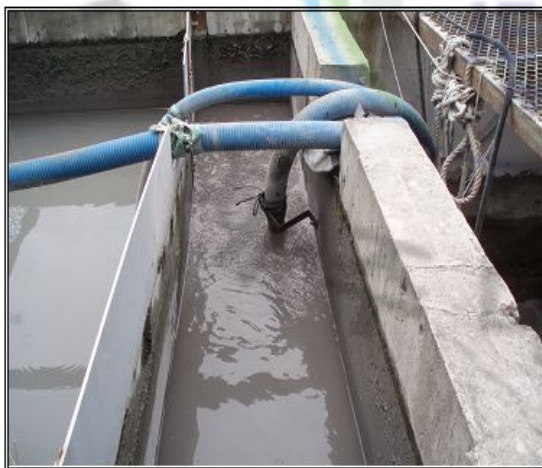
③ 1st Settling
