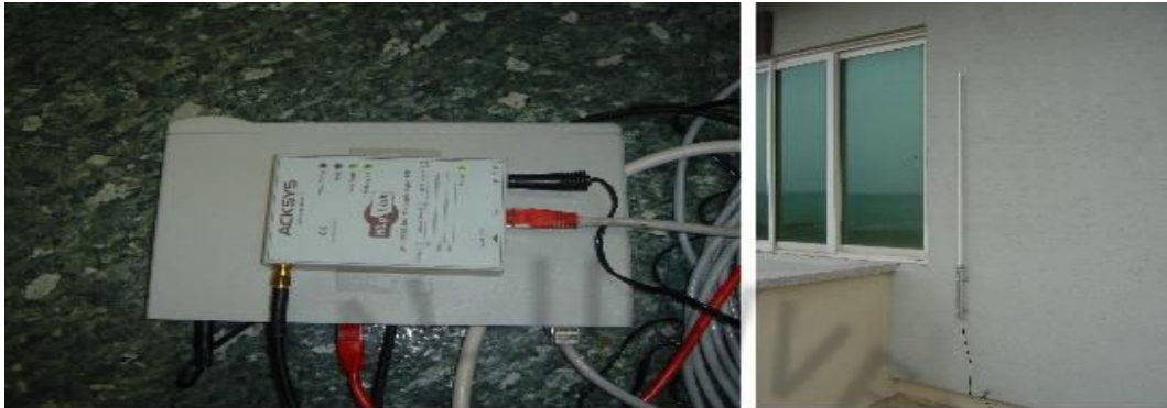
Fig. 14 AP(Access Point)and Exterior toward Antenna
