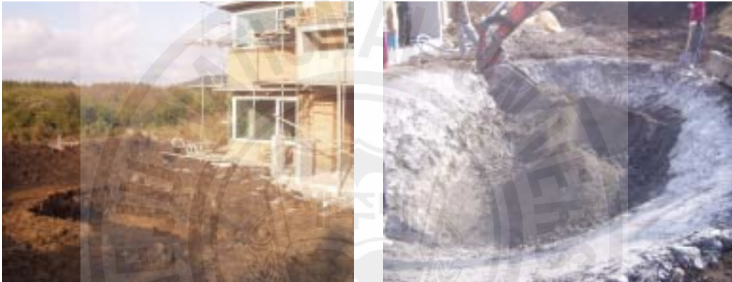
Fig. 6.10 The Pond Construction Process using Powered Basalt Sludge (The Pond Site, Mixing-1)
