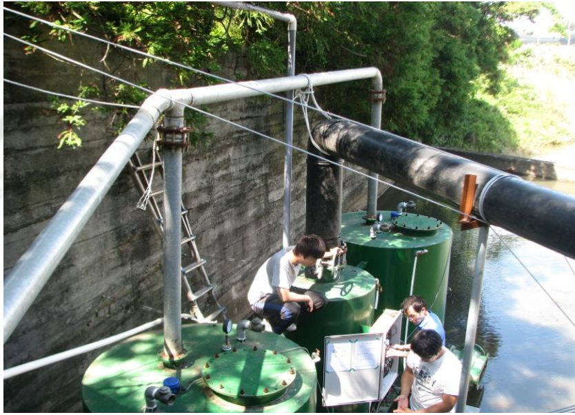
Fig. II-25 Check valve controller
