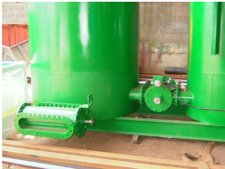
Fig. II-16 Installed motor and driving parts
