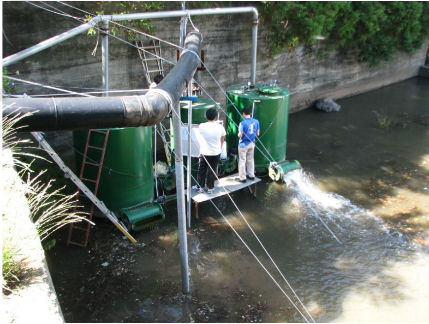
Fig. II-28 Water discharging situation at right chamber
