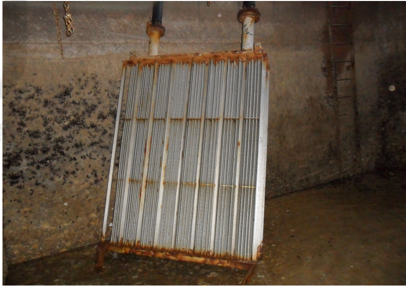
Fig. 11. Corrosion 1 of the heat retrieval system in the hot waste water tank used for the experiment.
