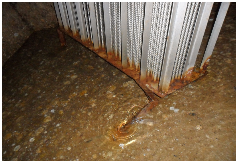
Fig. 12. Corrosion 2 of the heat retrieval system in the hot waste water tank used for the experiment.
