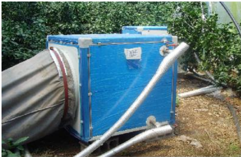
Fig. 9 The greenhouse heating/cooling system
