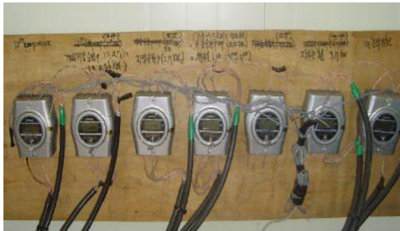
Fig. 11 The watt-hour meter
