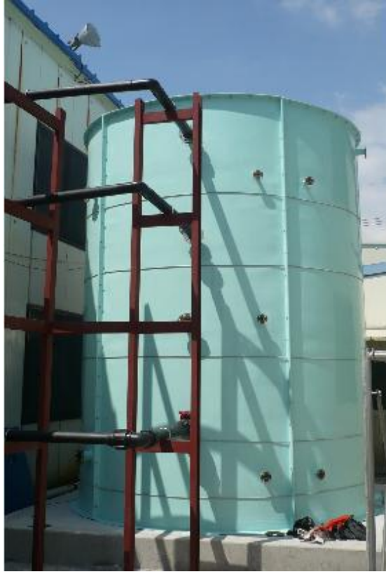
Fig. 8 The thermal storage tank of heat pump system
