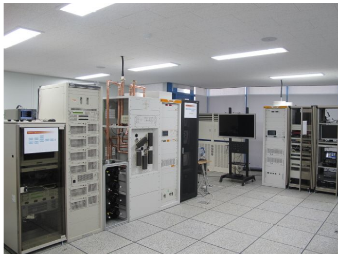
<Figure 14. TV broadcasting equipment>
