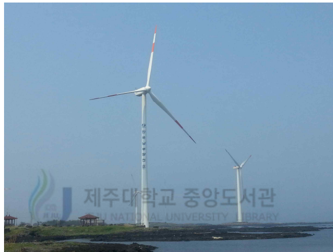
Fig. 6 View of WTG under test in Hankyeong wind farm
