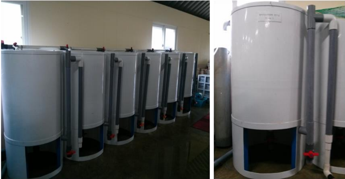
Figure 4. Feces collection tanks (Guelph system).
