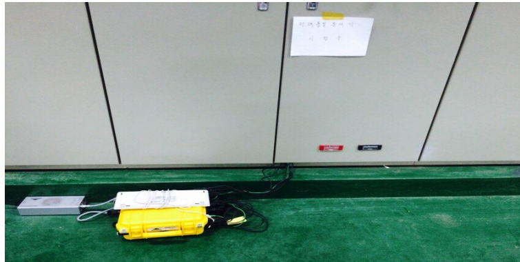
Fig. 1 Power quality analysis device connected 15.0 MW wind farm
