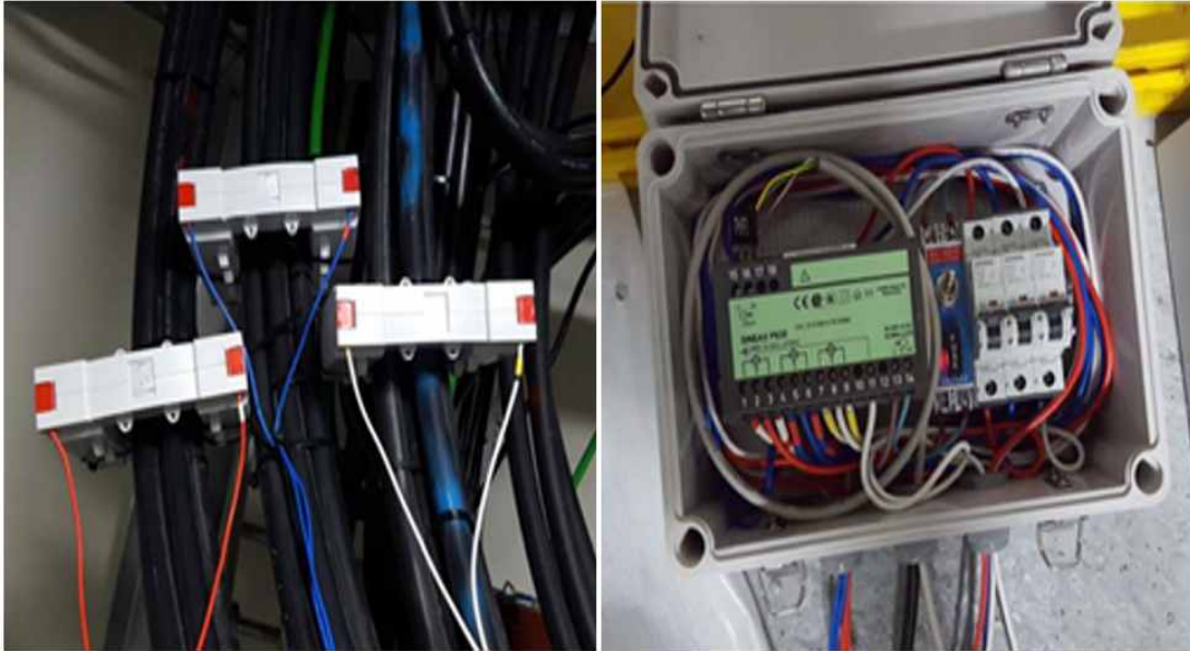
Fig. III-5 Current transformer and power transducer
