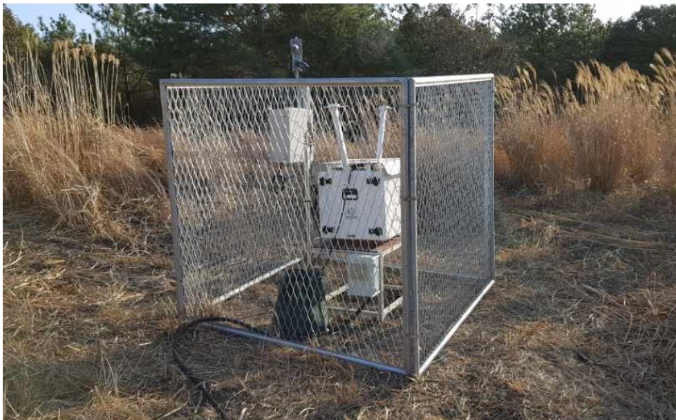
Fig. IV-10 Ground LiDAR installed at the Dongbok wind farm
