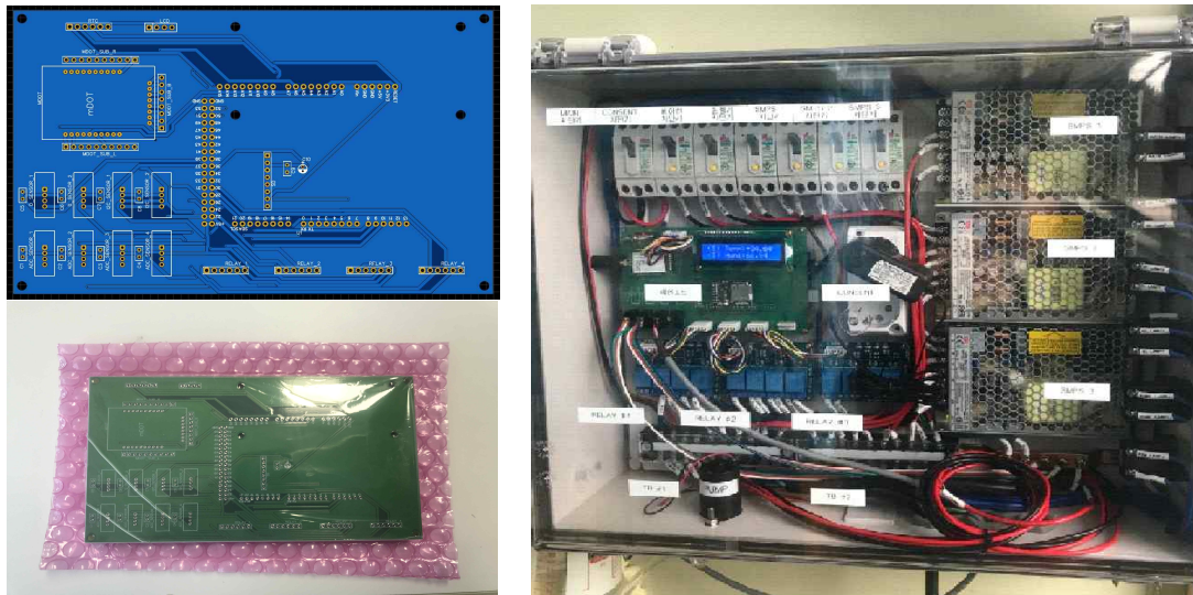
Fig. 3 Environmental control system controller
