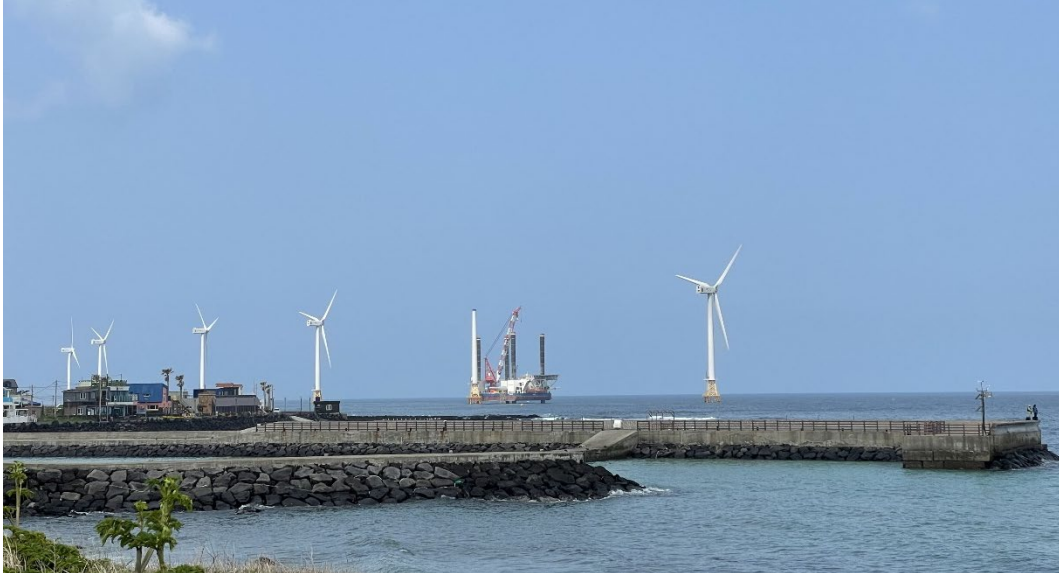
Figure 2 The wind turbine is being repaired at an offshore wind farm in Jeju.
