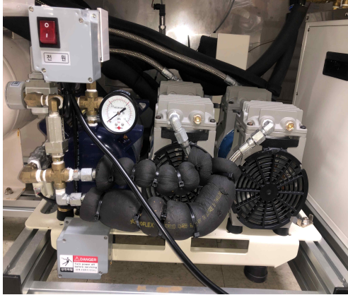
(a) Air compressor
