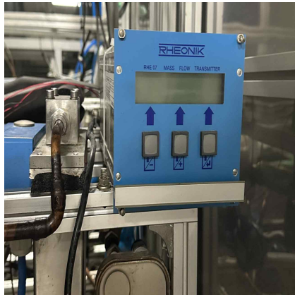
(c) Mass flow sensor (Refrigerant)
